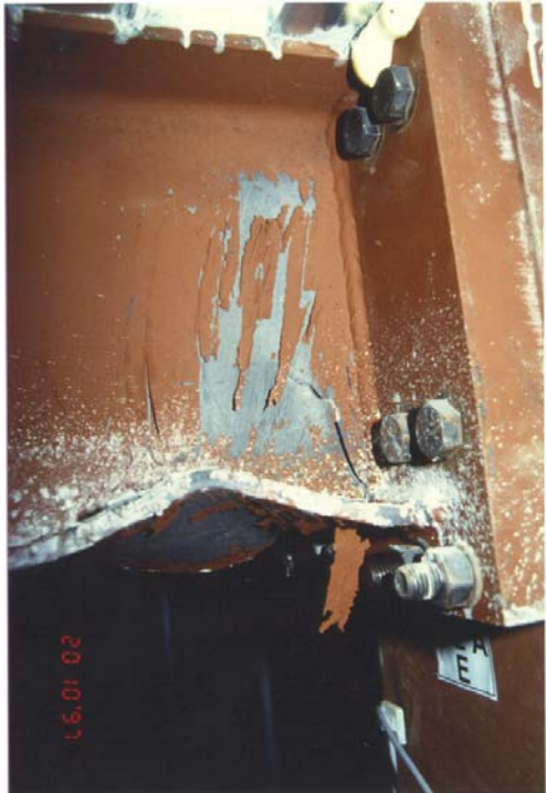
Picture 3.3.2. Buckling and fracture of the bottom flange
