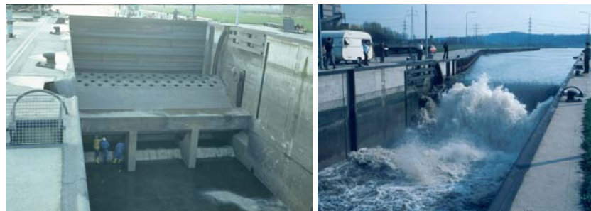
Figure. 15 - Upper gate at lock Lisdorf (D) during inspection and during a test for flood discharge
