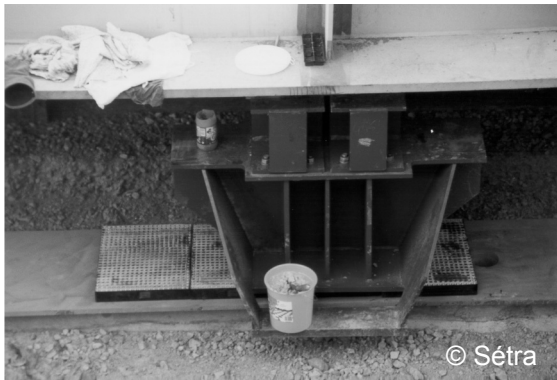
Figure 7-7: Sliding skate fixed under a vertical stiffener, Verrières viaduct near Millau, France, 2002.
