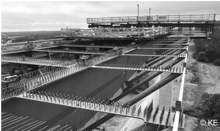
Figure 2-37: Small stands as support for formwork carriages “running on top”, valley bridge Reichenbach near Ilmenau, Germany, 2002.
