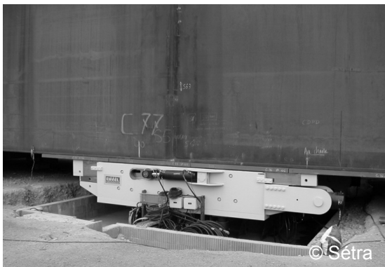
a) Jack system from the Millau viaduct (France)
