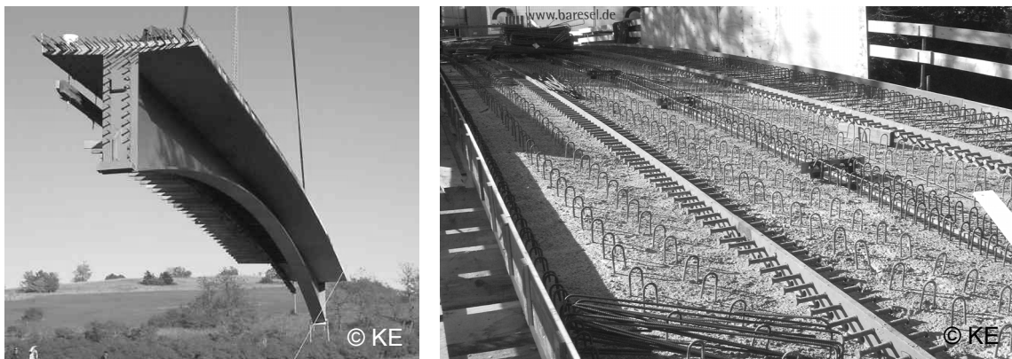
Figure 2-46: Erection of a prefabricated composite girder with horizontal studs near Münsingen, Germany.
