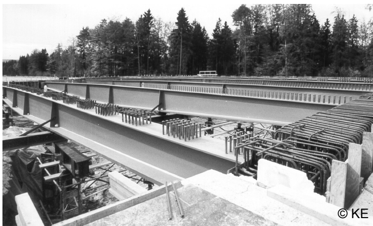
Figure 2-44: Erection of a bridge with steel girders and precast concrete elements near Ravensburg, Germany.
