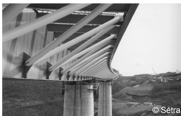
Figure 2-2: Box-girder bridge with edge beams supporting the deck. (Verrières viaduct near Millau, France, 2002).
