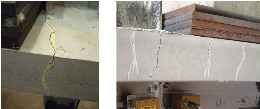
Figure III.40. Accentuated cracks in the vicinity of the external composite joints at the formation of the beam plastic mechanism
