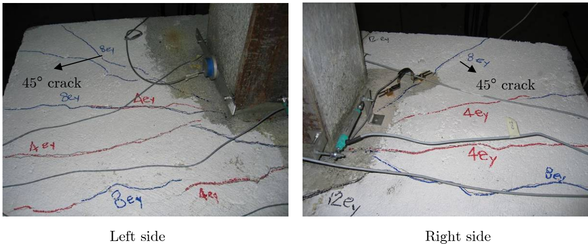
Figure II.23. Test 1 – Development of cracks in the composite slabs (at the end of the test)
