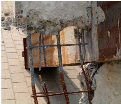
Figure II.35. Photo of the rebars behind the column at the end of the test
