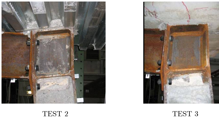
Figure II.27. Yielding of steel components at the end of TEST 2 & 3
