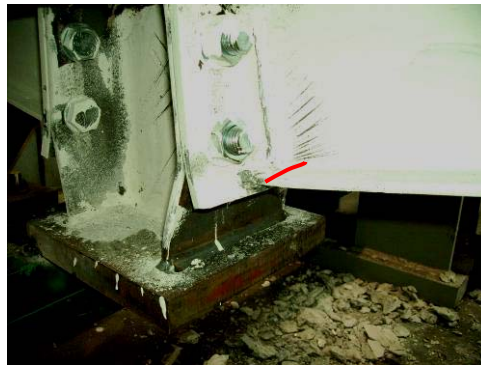
Figure III.49. Cracks in the welds between the IPE140 profile and the end-plate
