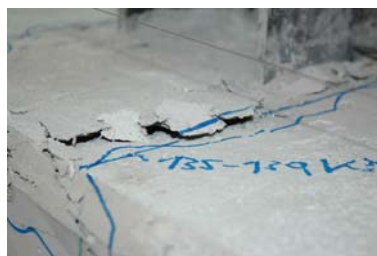
Figure III.67. Crushing of the concrete in the vicinity of the column
