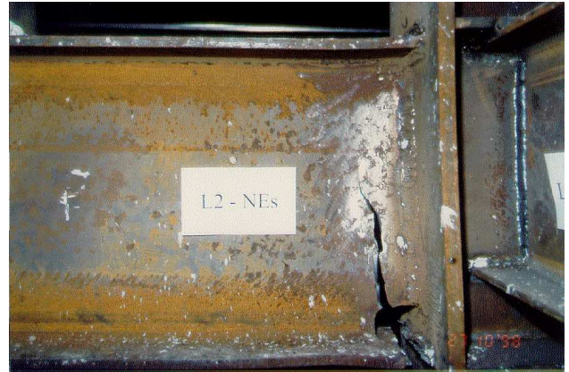
Figure 4: Example of a crack at a beam-to-column joint.
