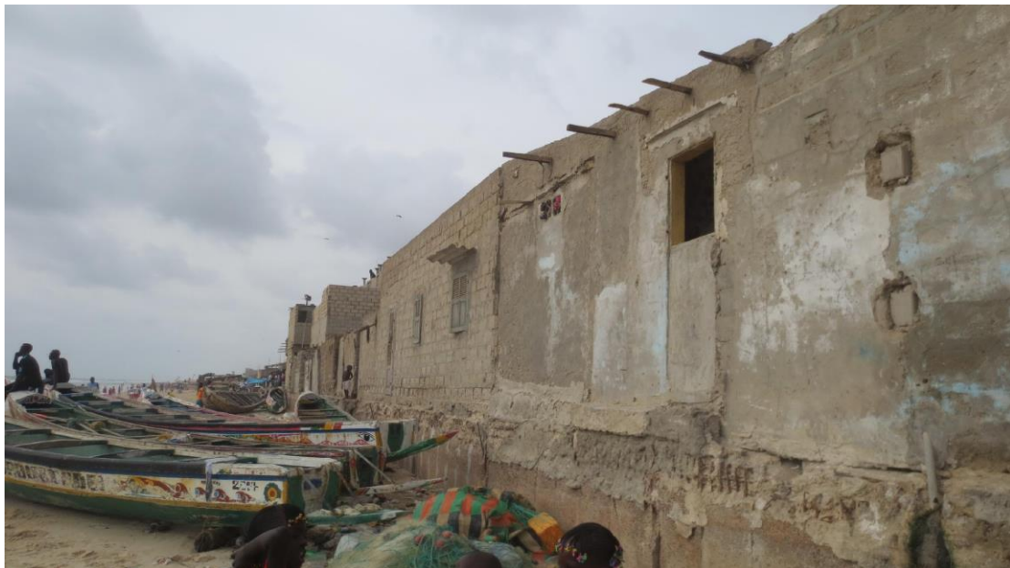
Figure 25 - Partially destroyed home in Guet Ndar, Saint-Louis 13
