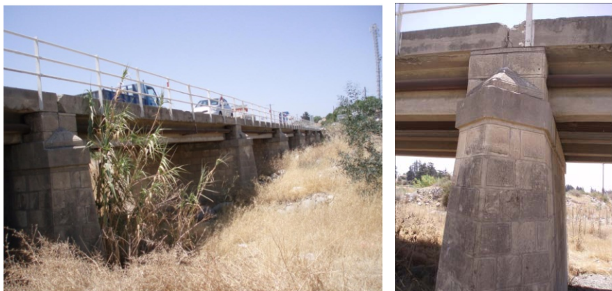
Figure 1. Typical photos of the existing bridge (Longitudinal view of the bridge and the pier).
