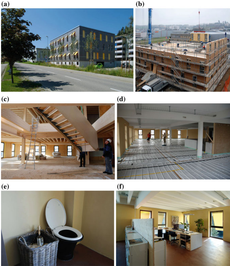
Fig. 6.2 a Simple building mass in a shape of a cube, Green Offices, Givisiez, Switzerland. b Prefabricated façade and floor units made from timber and blown-in cellulose flakes. c The four floors were constructed in 10 days with a high assembly precision. d Under ground floor heating coupled to a biomass heating system. e Waterless toilets connected to a compost unit in the basement resulted into 75% reduction of potable water use. f The open office interior and furniture is painted with VOC free paints
