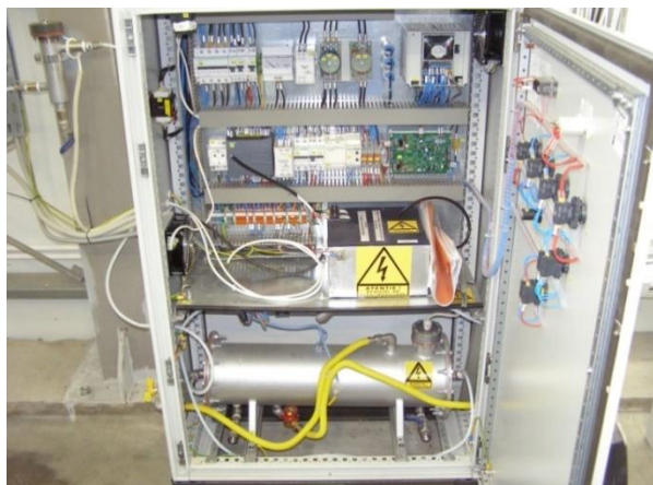
Figure 5. Ozone generator Source: Photo taken by authors
