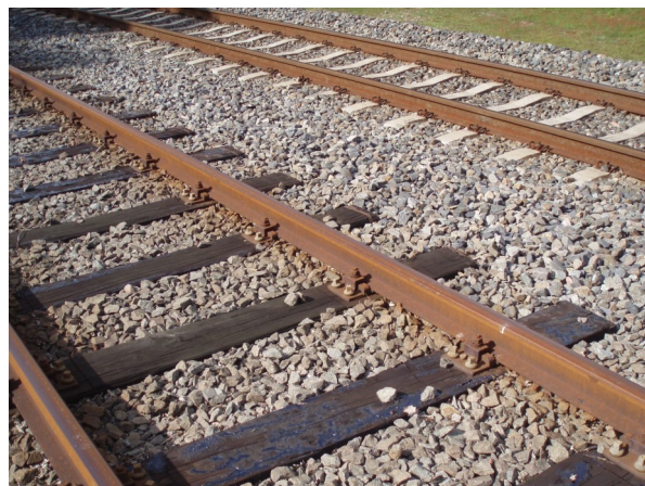
Figure 1. Coarse crushed stones of the ballast layer under a railway track. Picture by LooiNL, licensed under the Creative Commons Attribution-Share Alike 3.0 Unported license
