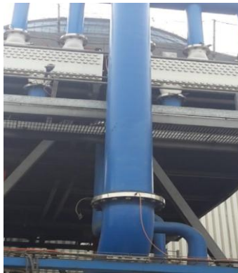
Fig. 3. View of the pipe connecting the condenser outlet to the pump inlet.
