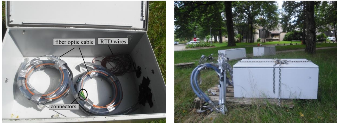
Figure 3.5 - Fiber optic cable loops (left) and metallic boxes (100 cm x 60 cm x 40 cm) for protection of the equipment (right)
