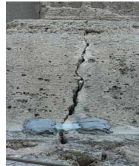
Images Showing the installation of the tell-tale device on the Taskisla building © Tania Ali Soomro
