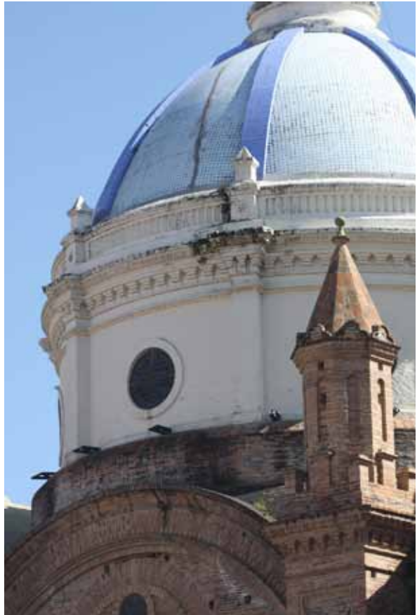
Crack on the small dome; Cathedral of Cuenca © Juan Diego Vele 2014
