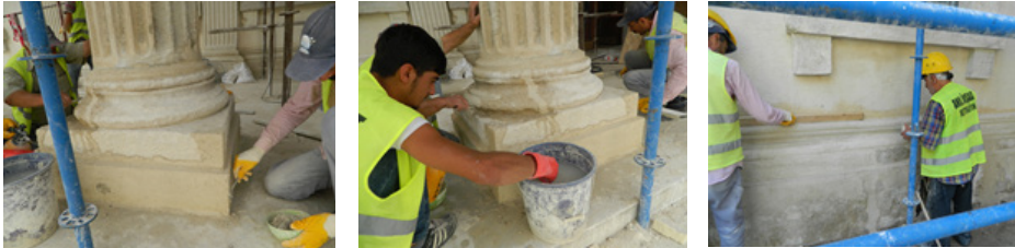
Images Showing the process of treatment of broken parts of the column base with lime mortar © Tania Ali Soomro
