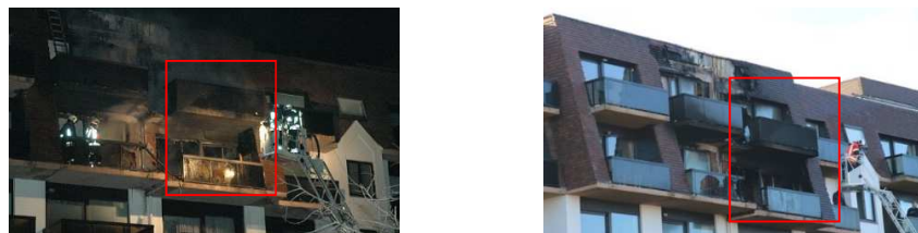
Figure 1. The façade and balconies affected by the fire are framed by the box
