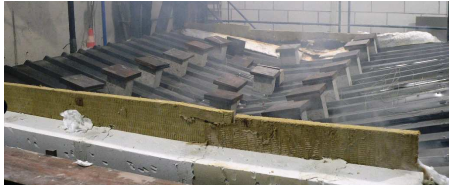
Fig. 10 Metal sandwich panel roof with mineral insulated core
