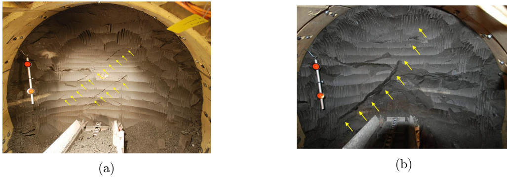
Figure 5.21: Fractures observed in the excavation front of Praclay gallery. (a) 0.5 m from the Connecting gallery. (b) 4 m from the Connecting gallery [Van Marcke and Bastiaens, 2010].
