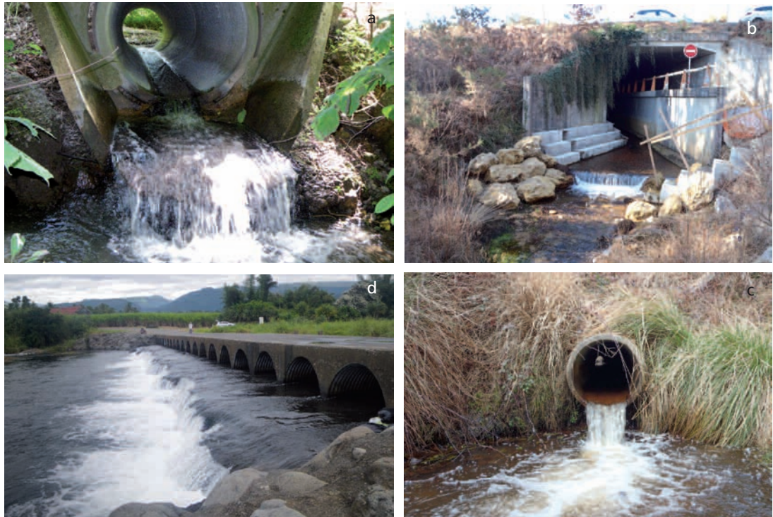
Examples of falls downstream of road structures.
