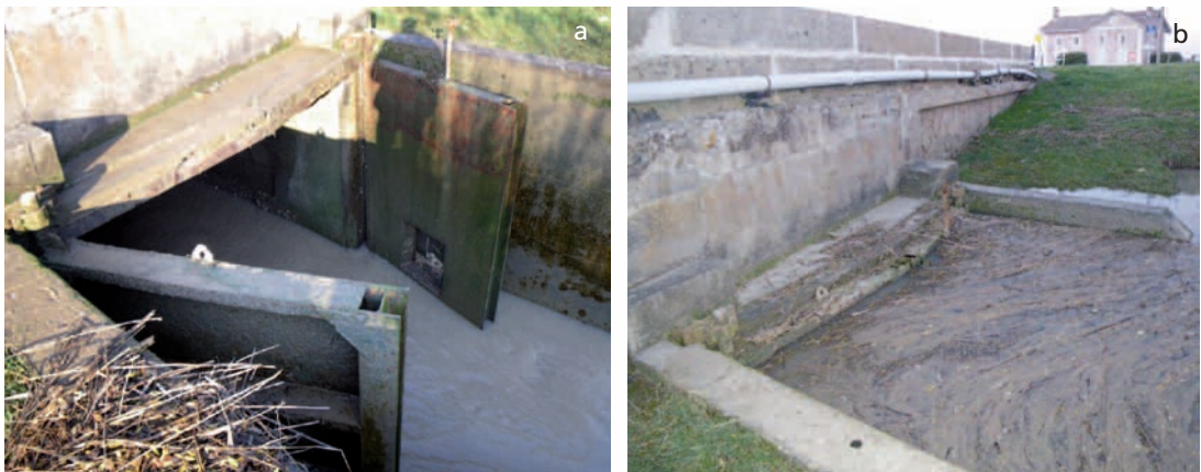
Example of tide gates on the Jalle de la Maréchale River in the Médoc region (near Bordeaux), (a) at low tide, (b) at high tide.
