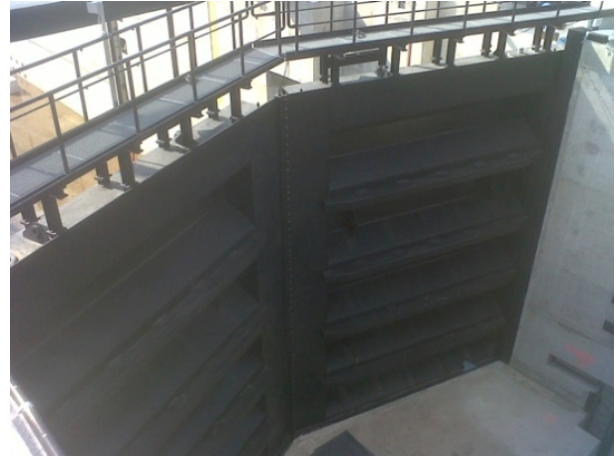
Figure 1. Mitre gates (Source INROS LACKNER AG).
