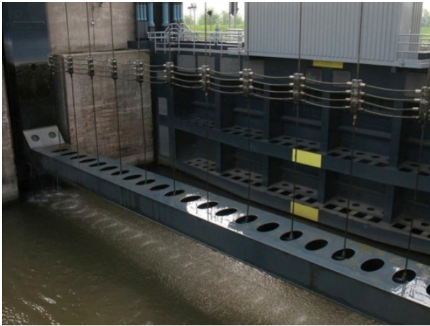
Figure 3. Movable ship arrestor net by a vertical lift gate during lifting, Bernhard Lock on the Amsterdam-Rhine Canal, The Netherlands (photo by R. Daniel)
