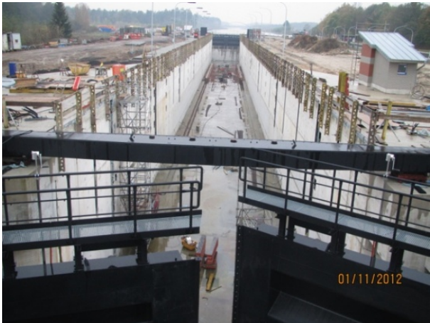
Figure 4. Shock absorber beam II (Old Navigation Lock Wusterwitz / Germany, photo by J. Ollero).
