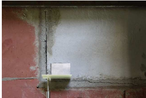
Figure 142 - Cracks near the lintel (after S6)
