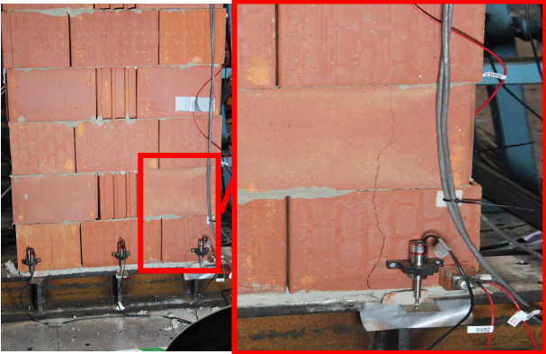
Figure 140 –Cracks in the “right” wall
