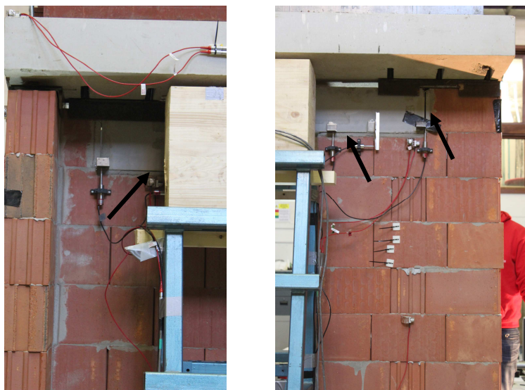
Figure 138 –Cracks at the interface between lintel and the walls
