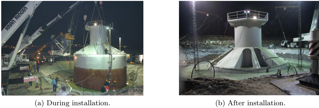
FIGURE 7.2: Installation of a prototype foundation at the test site of Frederikshavn, [Houlsby et al., 2005].
