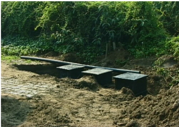
Fig.7 Water sewage treatments tanks
