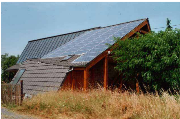
Fig.1 View of the PV and solar thermal roof of the building after the retrofit [4]
