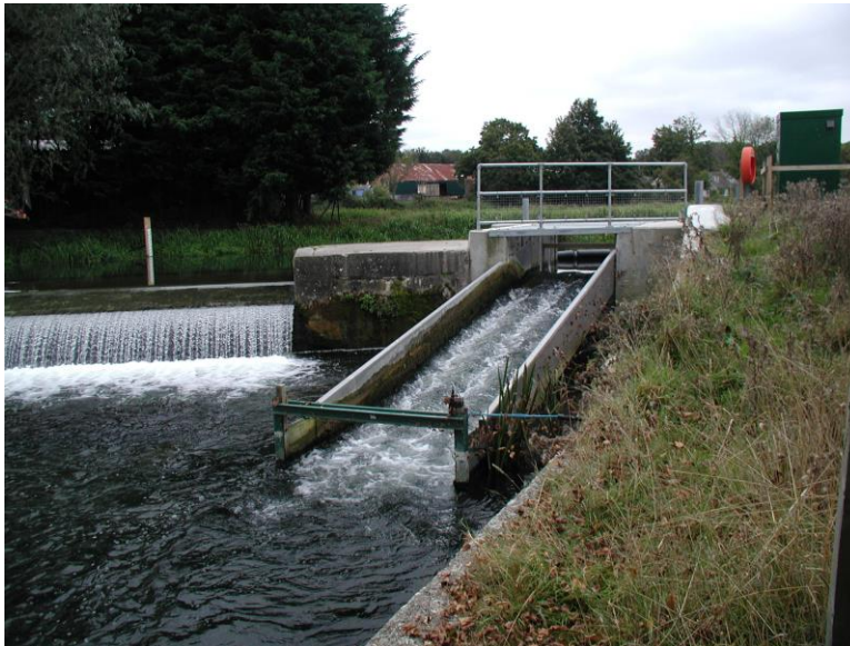
Example of fishpass at weir
