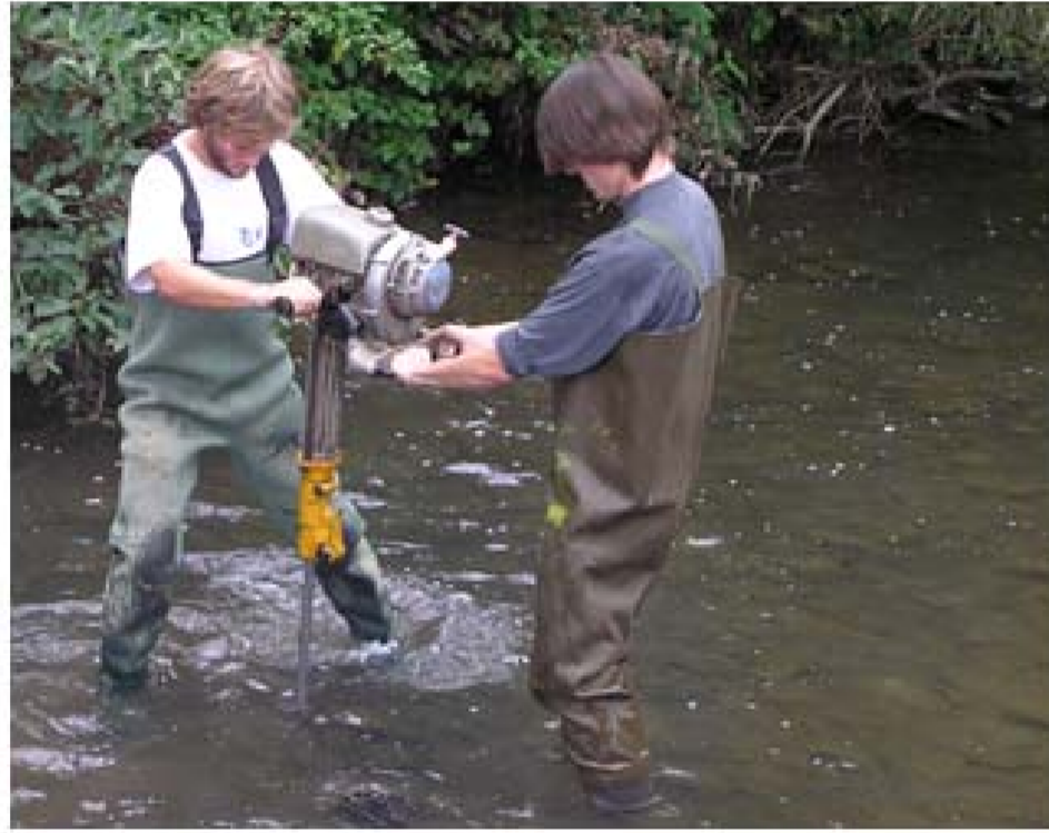
Pneumatic hammer used as a hand penetrometer to locate the contact gravel sheet / bedrock
