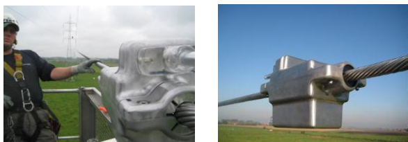
Fig 3: Installation of the smart grids sensor Ampacimon on a 150 kV line in the north of Belgium, near the North Sea.
