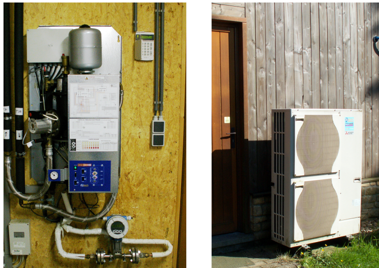
Figure 4.27: Installed vapour compression chiller internal (left) and external unit (right)
