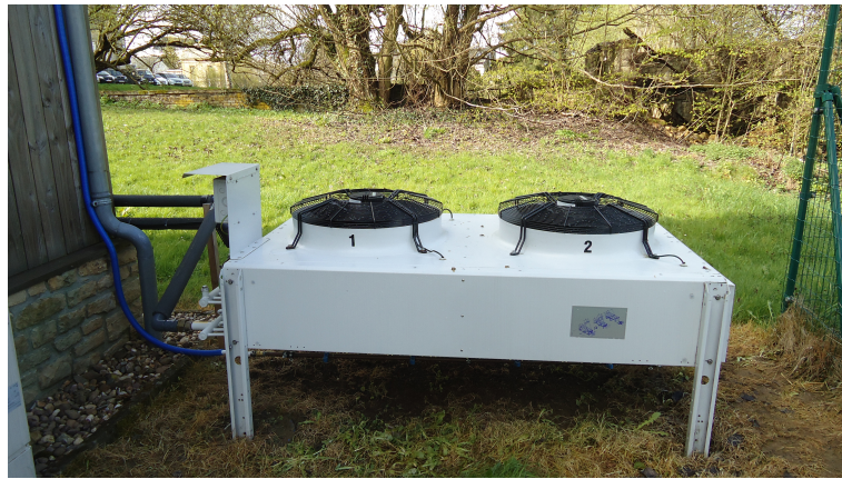
Figure 4.4: Dry cooling tower
