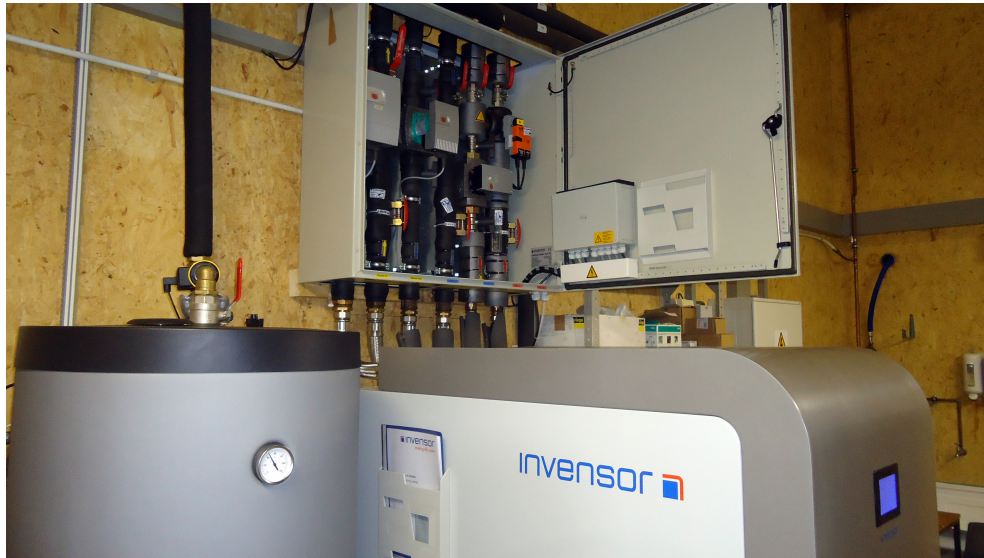
Figure 4.3: Installed adsorption cooling system with hot water tank (left), adsorption chiller (bottom) and hydraulics module (top)
