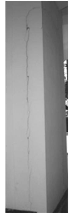
vertical cracking in a pile
