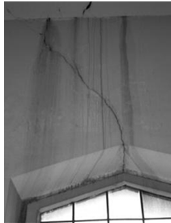
crack in the central part of the lintel
