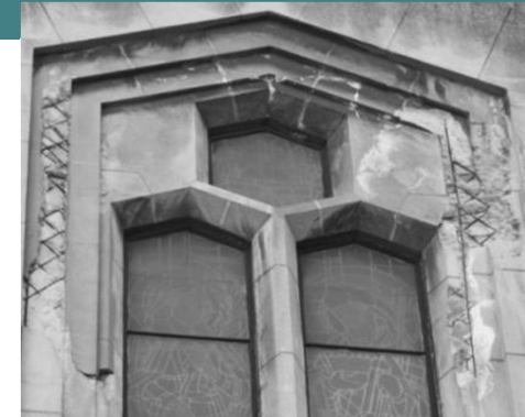
spalling, Saint-Vincent church, Liège
