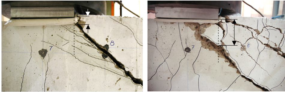
Figure 4.49 Critical loading zones after failure – specimens S0M (on the left) and S0C (on the right)
