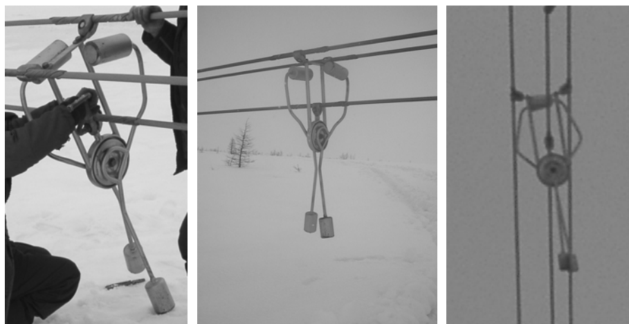
Fig. 2. Installation of the TDD antigalloping device on a Transmission Line: a) mounting on a bundle; b) the bundle before raising; c) the TDD is at a span of T/L
