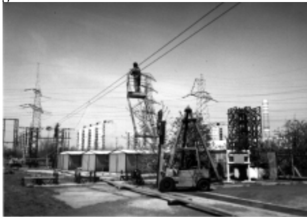
Figure 10.1 VEIKI test arrangement – 60 m span length – spacer at mid-span. The return path is on the ground.
